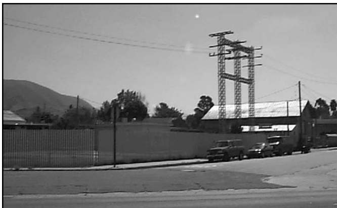
PG&E Substation at Walker and Pacific Streets
