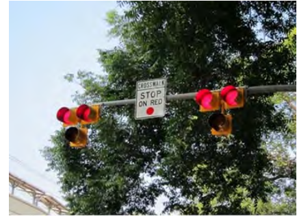
A pedestrian hybrid beacon (also known as the High intensity Activated crossWalk (or HAWK)) is a treatment that provides positive stop control in areas without the high pedestrian traffic volumes that typically warrant the installation of a signal
