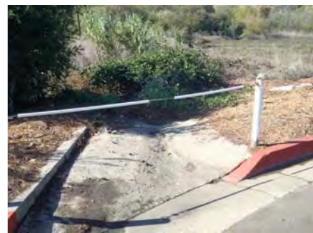
View of a spill way located at the southwest corner of the neighborhood located south Los Verdes #2. The area below the spill way and riparian area was wet during the survey. Note invasive giant reed located between the spill way and the riparian area.
