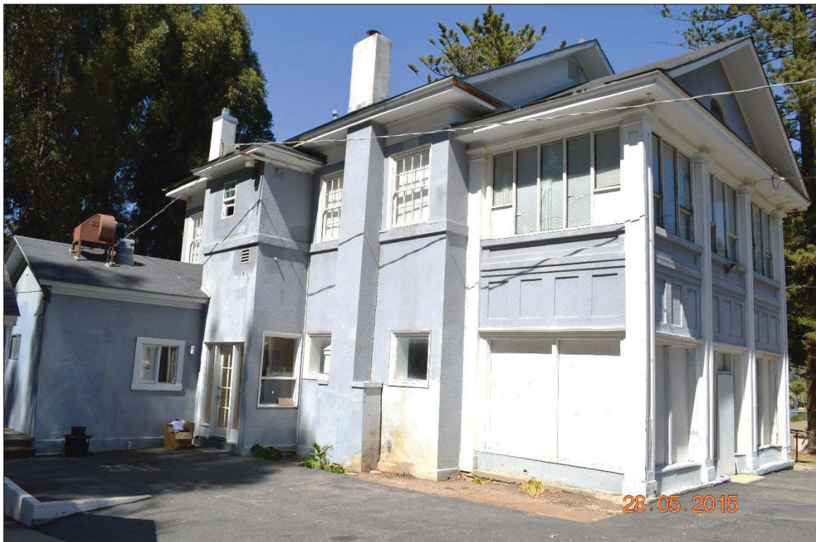
Figure 5-7 West (rear) façade of the Sandford House with a single-story addition on the northwest corner of the building.
