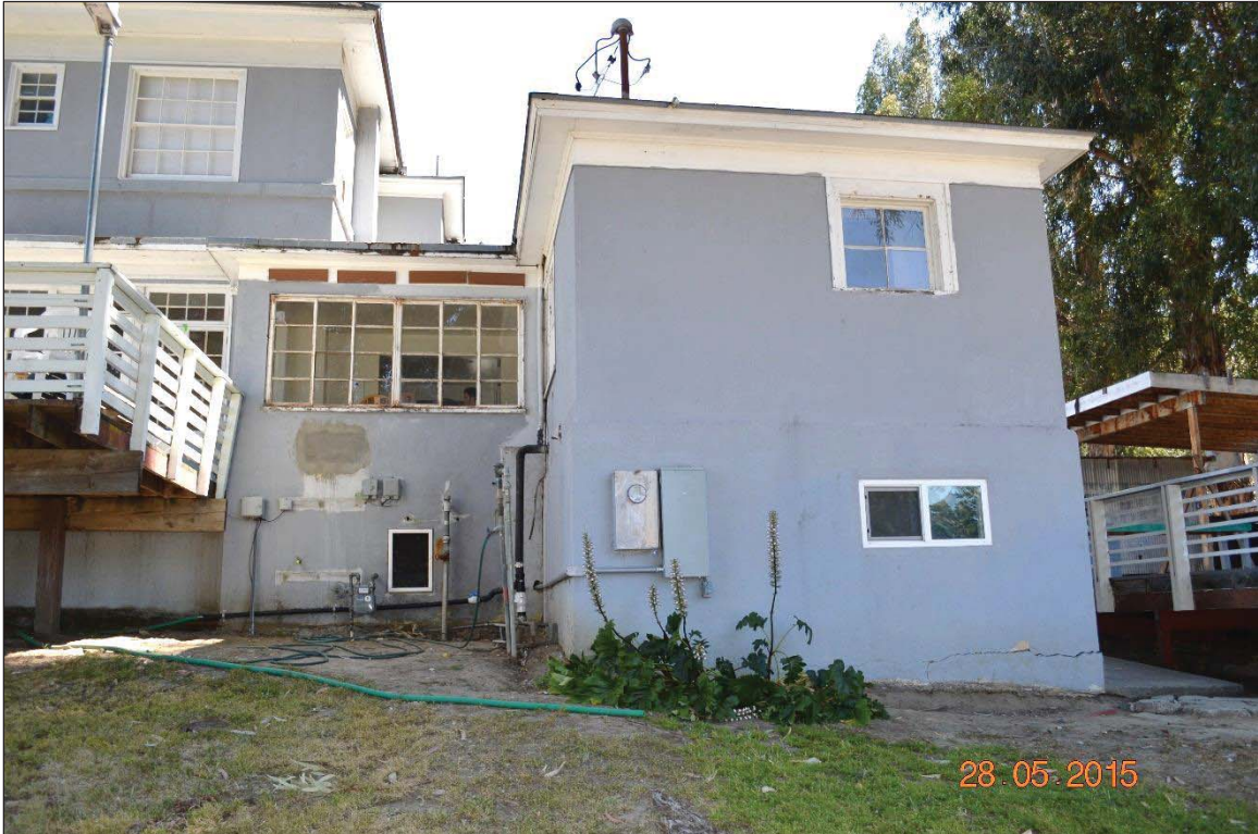
Figure 5-9 North façade of two-story addition to the Sandford House; the single-story addition is attached to the south.
