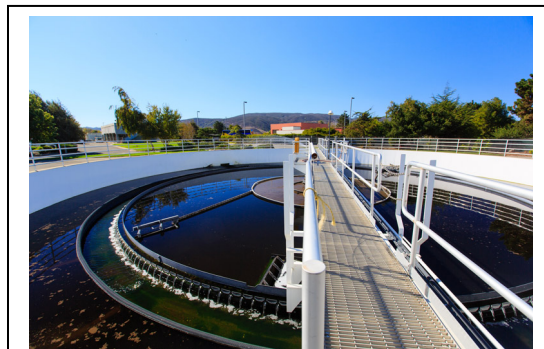
The WRRF removes solids, reduces the amount of nutrients, and eliminates bacteria in the treated wastewater before it is discharged to San Luis Obispo Creek.
