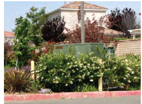
Plant material was used to screen this mechanical equipment from view
