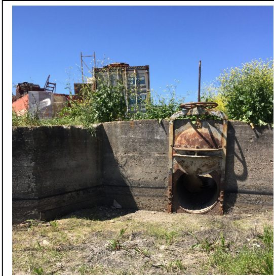
To the west of the Chevron Tank Farm property is an operational gate valve, which regulates the flow of Tank Farm Creek.
