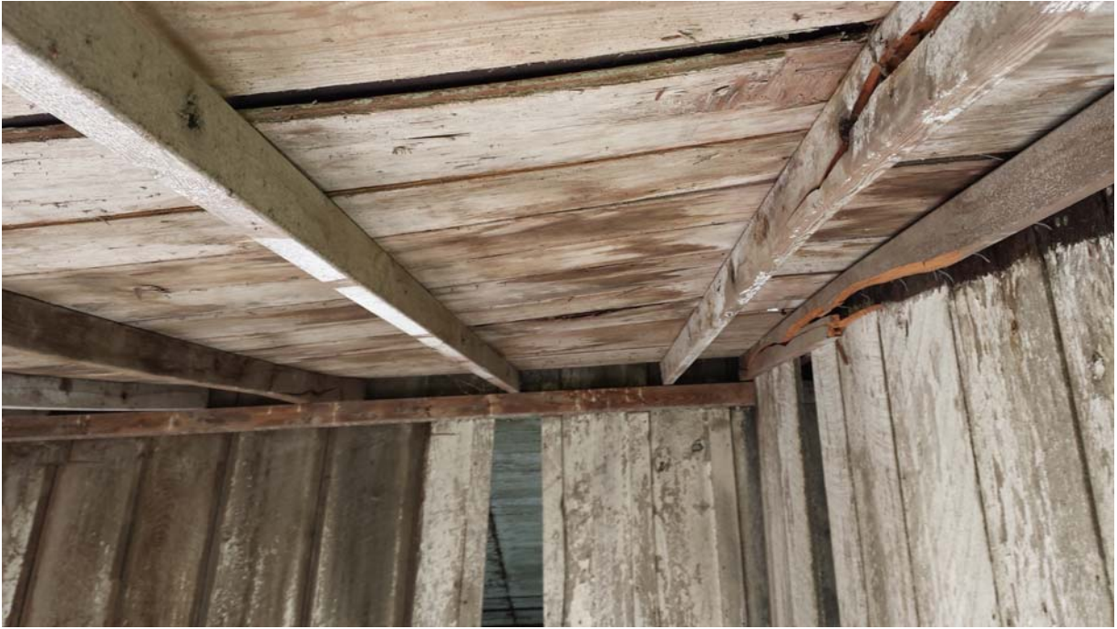
Figure 16 – Deterioration of Creamery House
