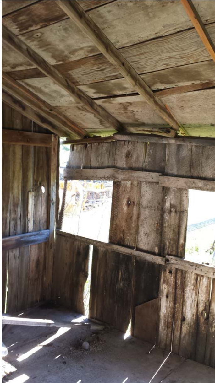
Figure 18 – Deterioration of Creamery House
