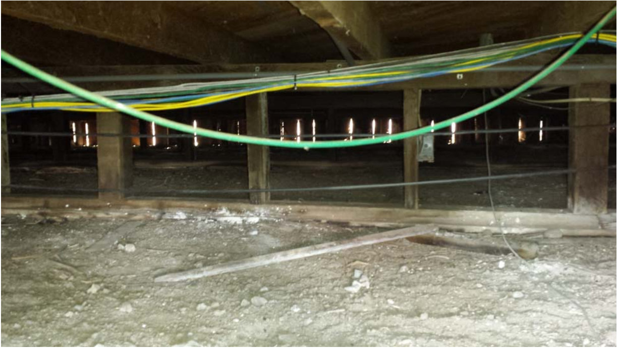
Figure 3 – Unbraced wood cripple wall with redwood sill
