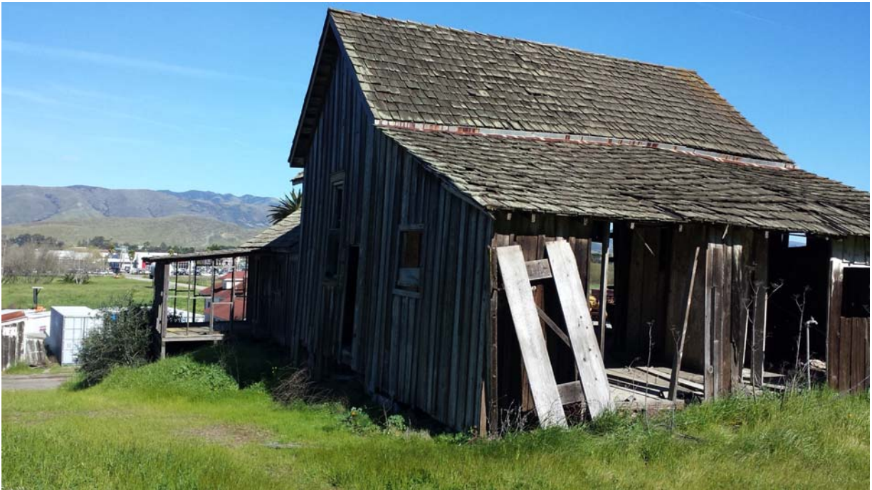
Figure 15 – Deterioration of Creamery House
