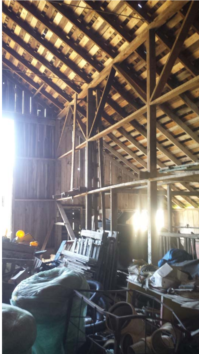
Figure 7 – Lack of wood bracing at main western entrance to the Dairy Barn
