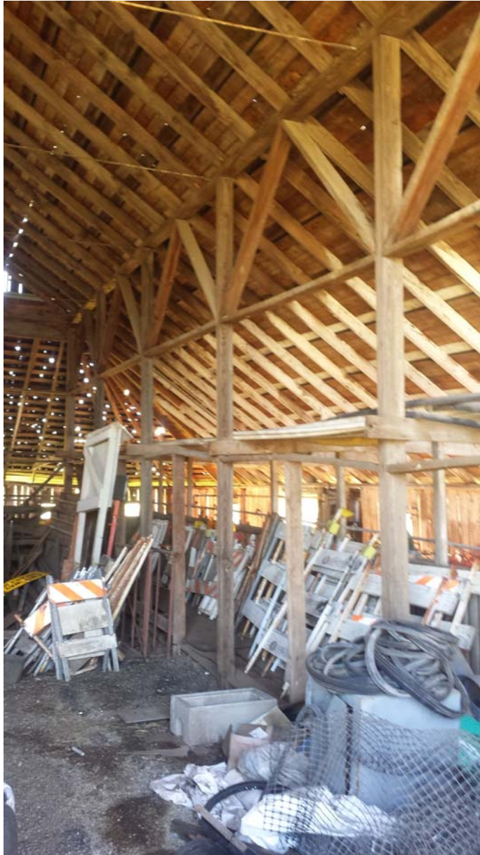
Figure 9 – Interior Dairy Barn posts bearing on soil
