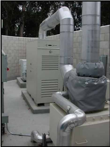
Natural gas co-generation equipment at Sinsheimer Pool saves City residents energy and money by heating pool water while producing additional energy to power lights, pumps and other electrical equipment
