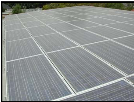
Roof-mounted photovoltaic panels produce electricity which helps meet the Ludwick Recreation Center's energy needs
