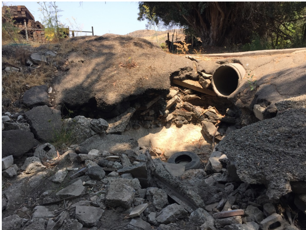
Photograph 10. The downstream (southern) end of the existing crossing over Acacia Creek (August 8, 2018).
