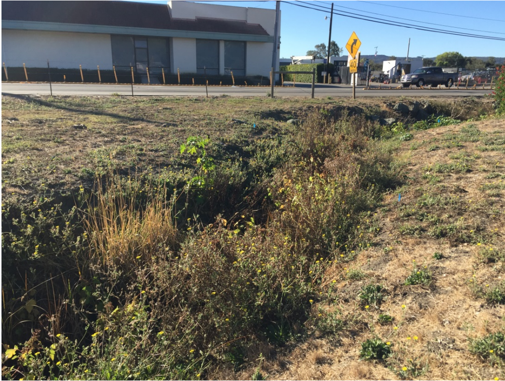
Photograph 3. Orcutt Creek in southeastern corner of Study Area, upstream of the culverts beneath Tank Farm Road (October 24, 2017).
