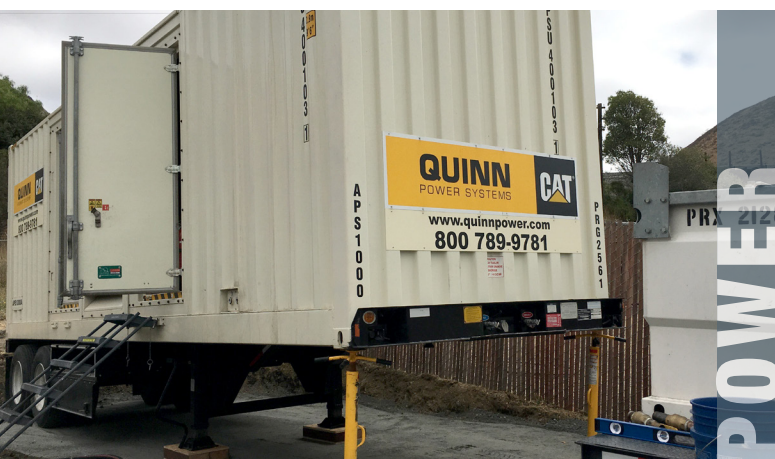
Rental Generator at the City's Stenner Canyon Water Treatment Plant.
