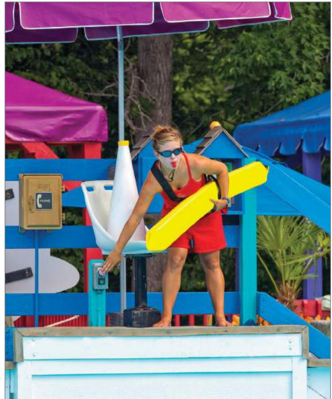
Figure 5-6 | Pushing the emergency stop (E-stop) button stops waves at a wave pool.
