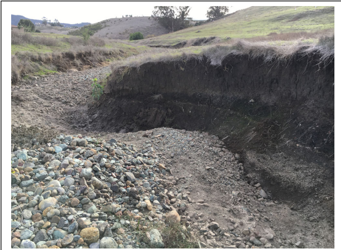
Froom Creek traverses the Project site within a narrow channel composed of rock, gravel, and sand. Evidence of eroded, undercut banks from high-velocity flows was observed onsite (January 2018)
