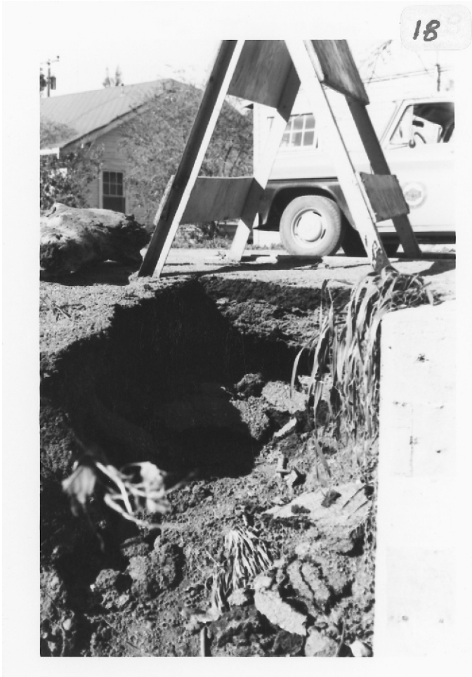
Wash out at Nipomo and Stenner Creek
