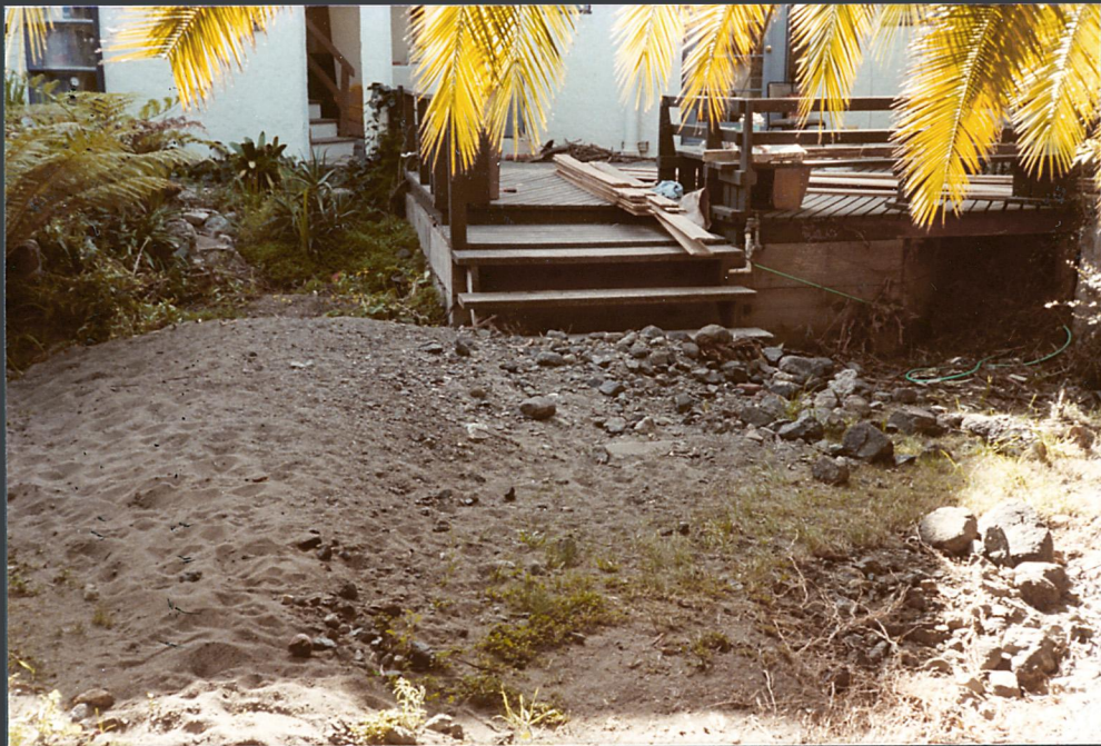
26. 1822 Johnson Water jumped channel and flooded basement
