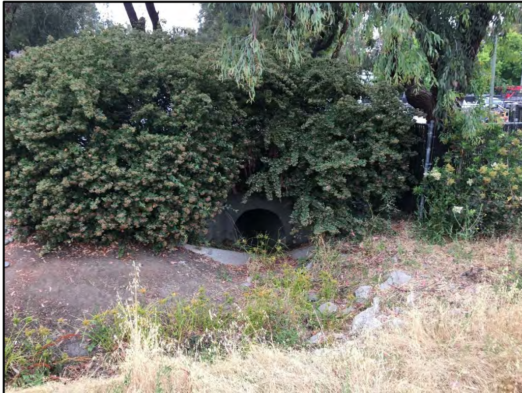
Photo 6. 48-inch box culvert that extends under Fiero Lane and outlets to Acacia Creek, (Aspect: North).
