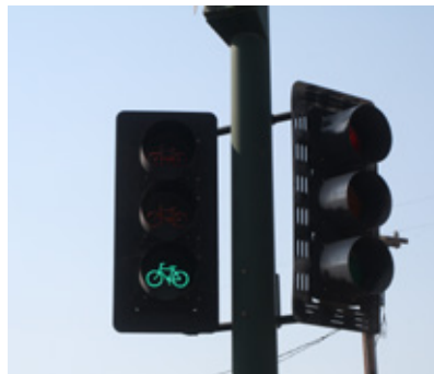
BICYCLE TRAFFIC SIGNAL
