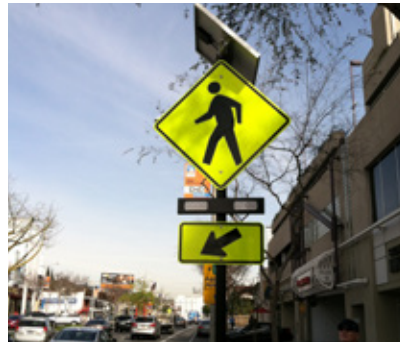
RECTANGULAR RAPID FLASHING BEACON (RRFB)
