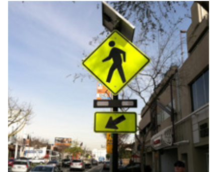
RECTANGULAR RAPID FLASHING BEACON
