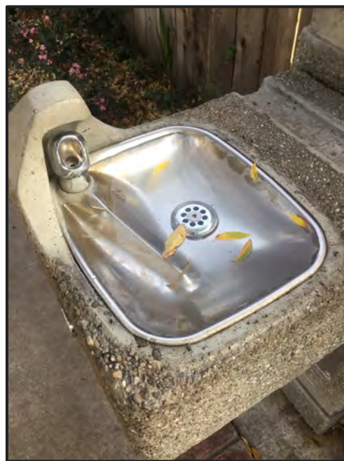
Figure 1a. Clogged drinking fountain (rated 2)
