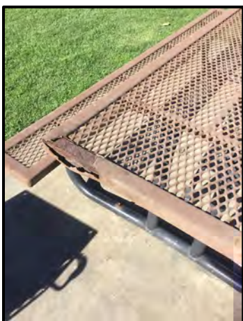
Figure 15b. Picnic Table with exposed metal
