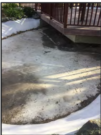
Figure 3b. Drained water body (rated 3)
