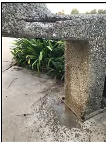
Figure 14b. Leaking cement drinking fountain
