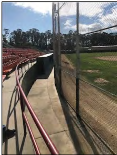
Figure 24e. Potentially dangerous railing for children
