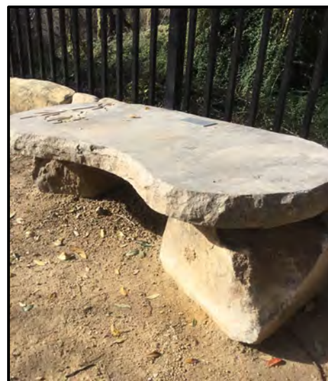
Figure 8a. Bench surface not properly secured to legs (rated 1)
