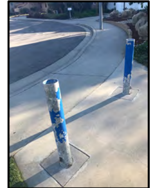
Figure 14a. Paint chipping on bollards
