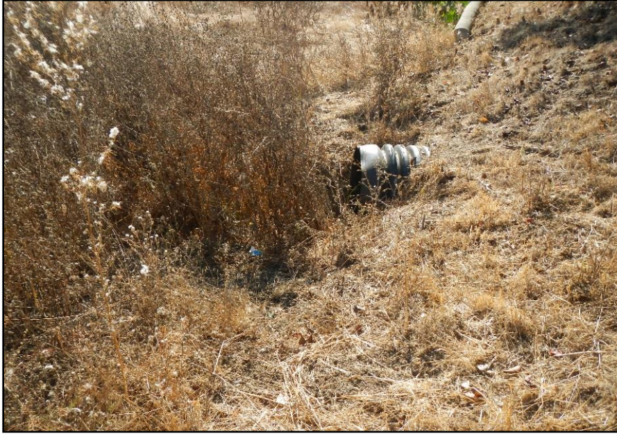
Photo 7. Culvert in the northwest corner of the survey area where the drainage discharges from the site (11-11-19).
