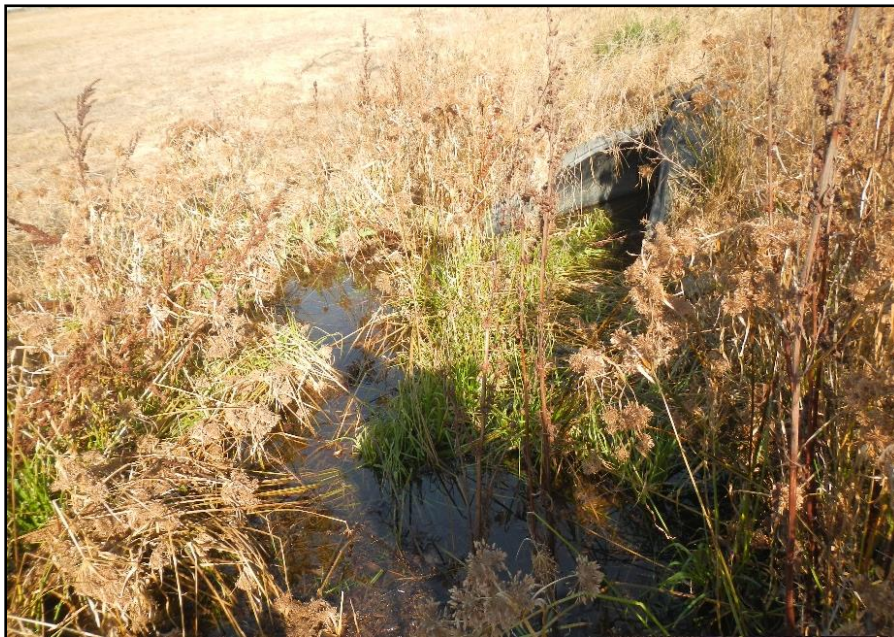
Photo 6. The culvert under Aero Drive where the drainage enters the survey area. There was water ponded at the outlet. Water appears to be from irrigation of the bioswale plantings in the parking lot south of Aero Drive (9-30-19).
