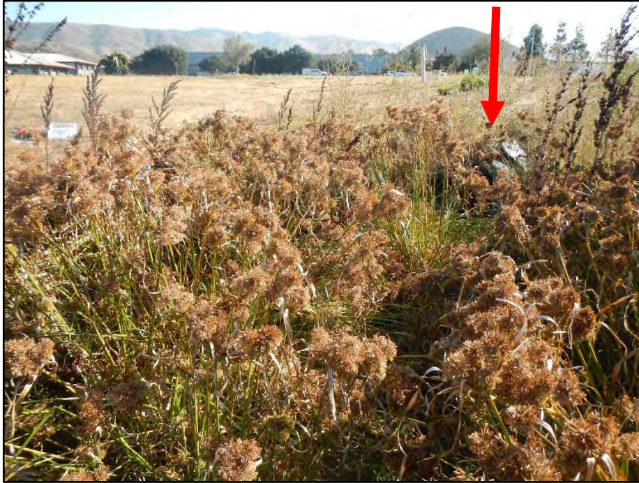
Photo 3. View of culvert under Aero Drive (red arrow) where drainage enters the survey area, aspect northeast (10-03-19).
