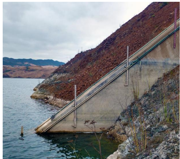
Whale Rock Reservoir Level Gauge.
