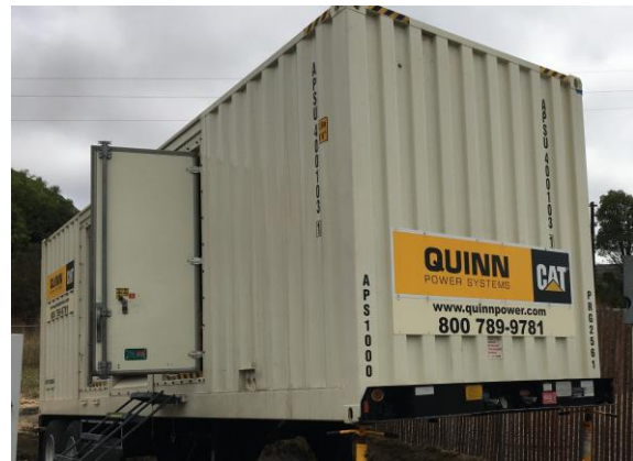
Temporary Generator and the City's Stenner Canyon Water Treatment Plant.
