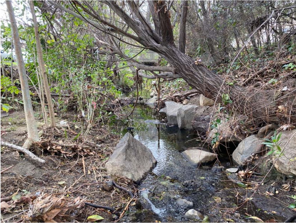
Photo 5. Some parts of the channel may have been armored during construction in this area. Flowing water was present and it ranged from 2 to 6 inches deep.
