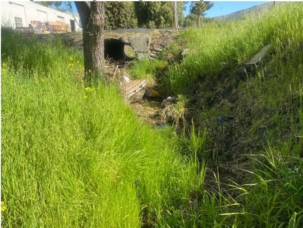
Photo 10. View from within the channel looking upstream at the culvert, with concrete slope protection around it. The tree is the same red willow as in Photo 9.
