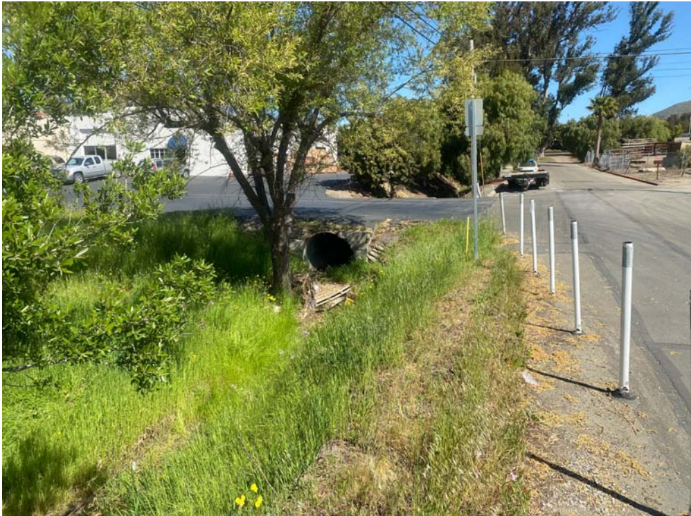
Photo 6. View from the eastern property boundary looking north. A portion of the paved driveway and culvert fall within the parcel boundary. The drainage enters the property from this culvert and the upstream area is a ditch along McMillan Avenue seen in the distance. Two Cambria morning glory plants were seen at the base of the sign in this photo.
