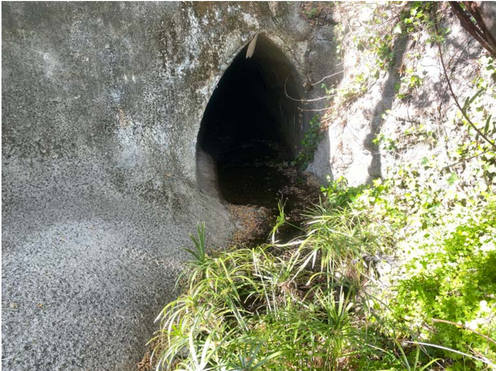
Photo 14. View of the culvert on the downstream side of the drainage with concrete slope protection. From this point the drainage runs under an industrial complex offsite.
