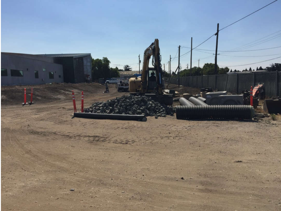
Photograph 7. View of construction associated with new development along Prado Road, facing east.
