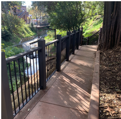
Mission plaza railing was replaced in 2021-22 as part of the Mission Plaza Maintenance Improvements Project.
