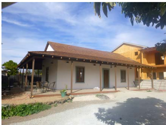
Mancilla/Freitas Adobe, 868 Chorro Street, c. 1800-1850. Photo of rehabilitation 2014; source City of San Luis Obispo.
