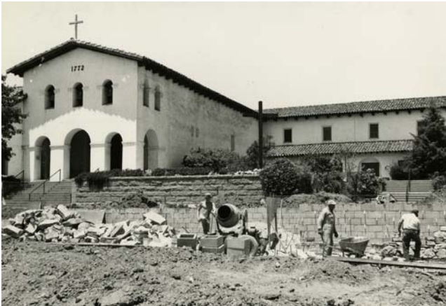
Mission Plaza during construction, 1970. Source: Cal Poly San Luis Obispo, Special Collections.
