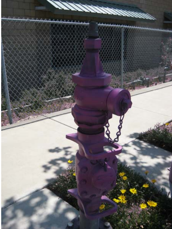
Recycled water is available from four wharf head s around the City
