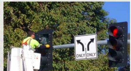
Traffic Signal & Street Lights
