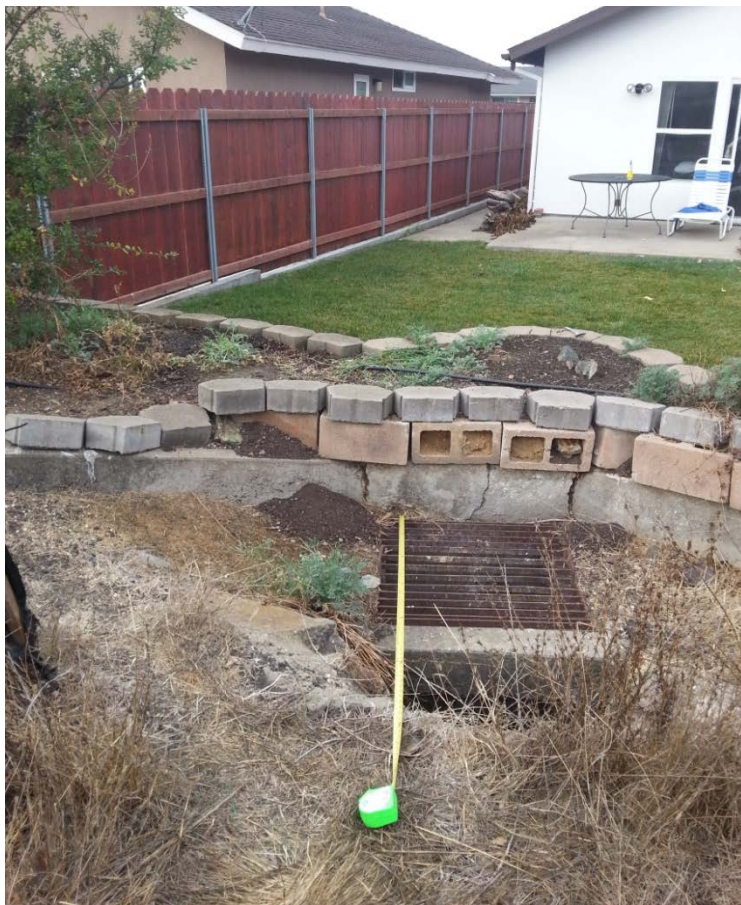
Photo 4. Drop inlet a downstream terminus of swale. Stormwater flows through pipes under the house to Calle Jazmin.
