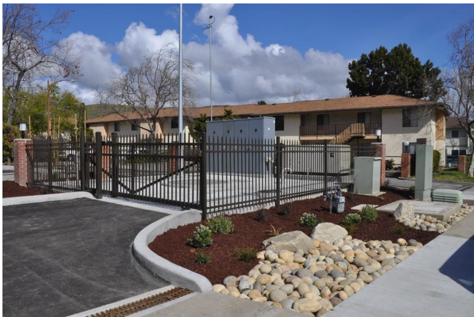
Margarita Lift Station, 2019.
