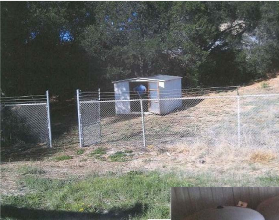
Reservoir Canyon Pump Station - Exterior and Interior
