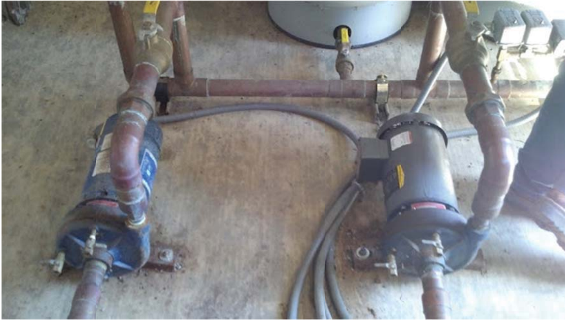
Reservoir Canyon Pump Station - Interior
