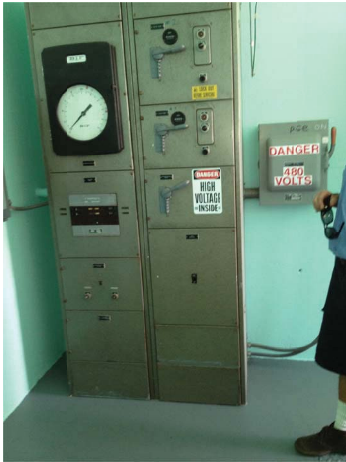
McCollum Pump Station - Interior
