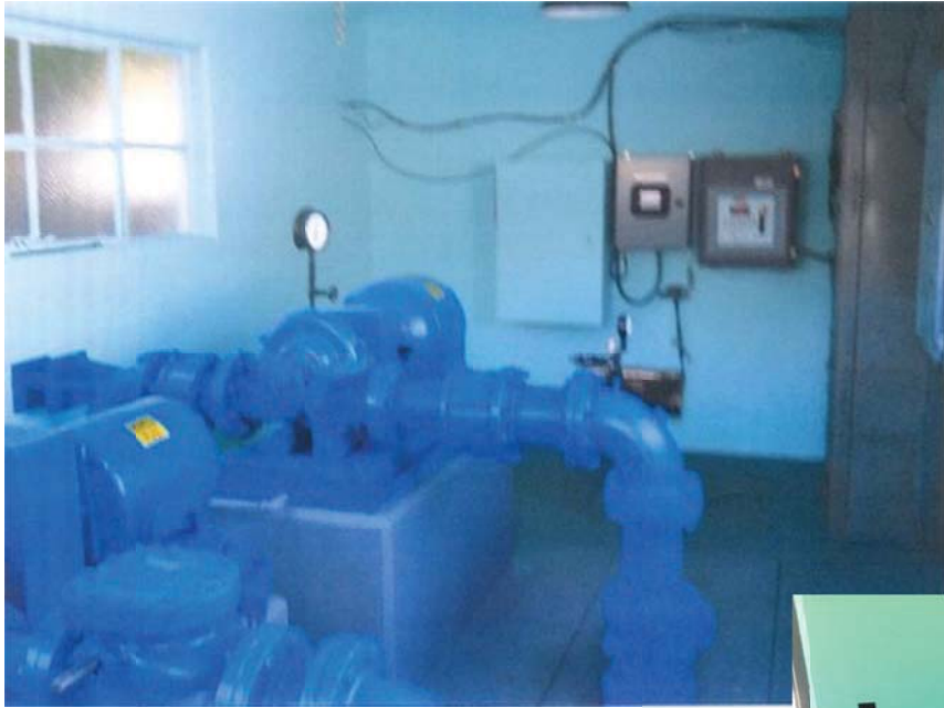
McCollum Pump Station - Interior
