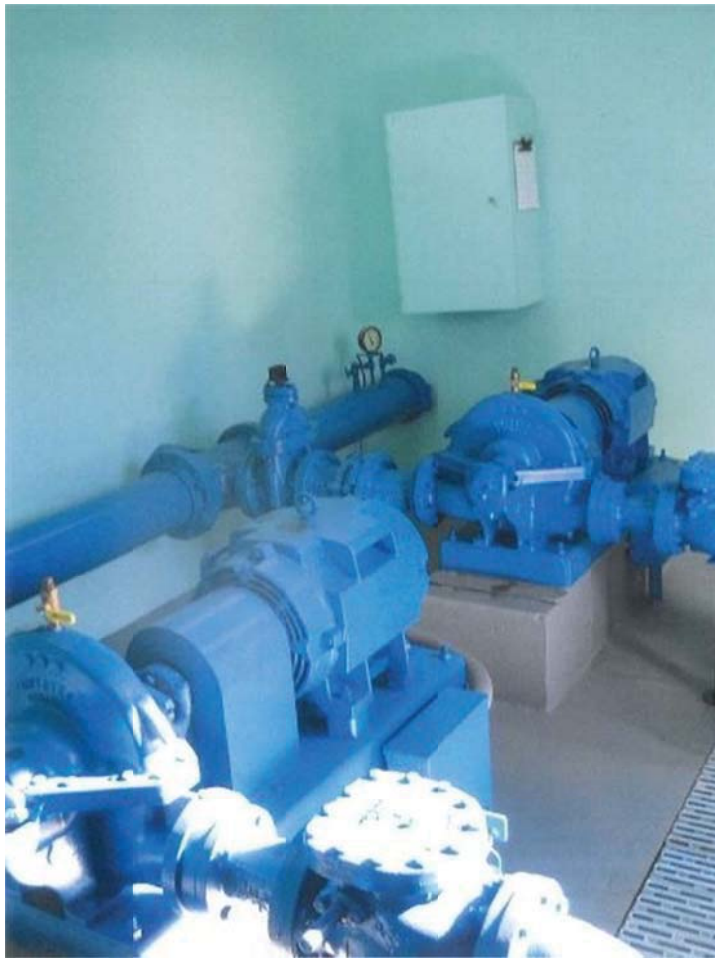
Bressi Pump Station - Interior
